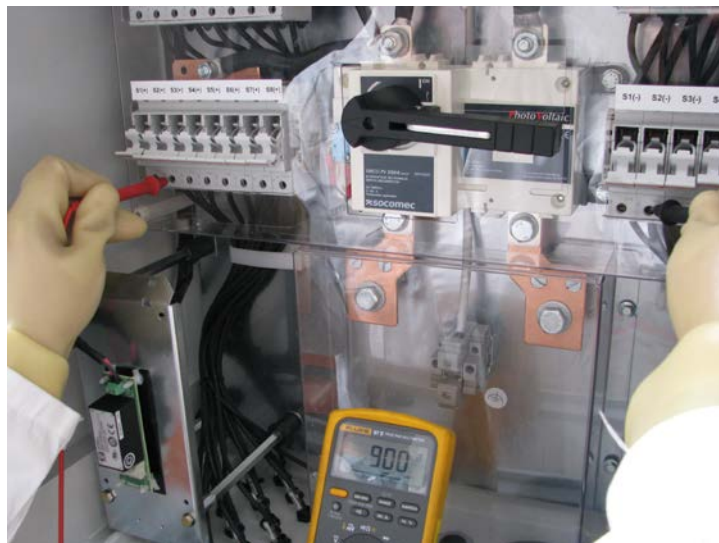
Figure 22: Voltage measurement points (string check 2: correct mounting)
