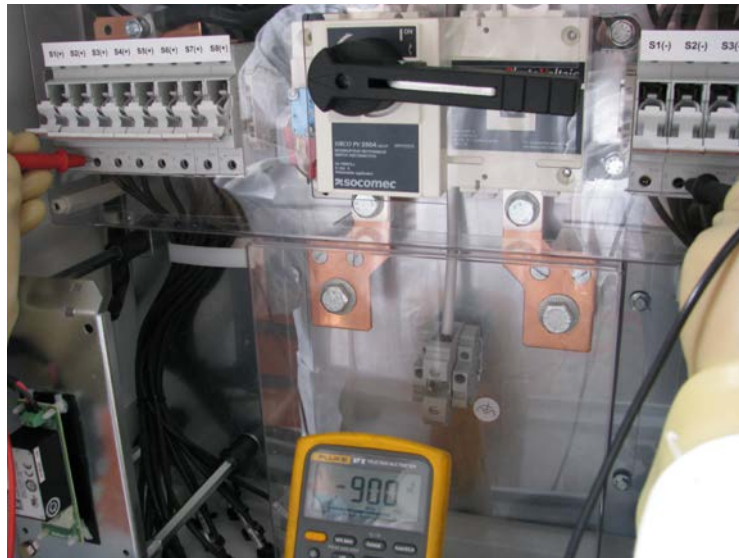
Figure 23: Voltage measurement points (string check 2: string mismatch!!!)
